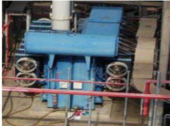
Gambar 3.8 BBT ( Auxiliary Transformer ) 21 kV / 10,5 kV
