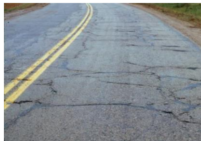
Gambar 2.12 Retak blok ( block cracking ) (Sumber: Google Image )
