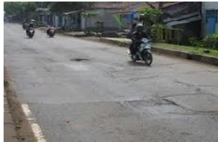
Gambar 2.13 Retak slip ( slippage cracking ) (Sumber: Google Image )
