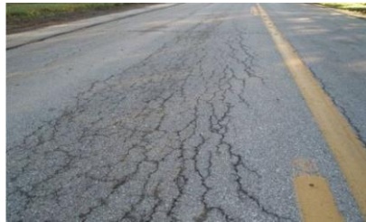
Gambar 2.9 Retak melintang ( transverse cracks ) (Sumber: Google Image )
