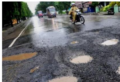
Gambar 2.16 Lubang ( potholes ) (Sumber: Google Image )
