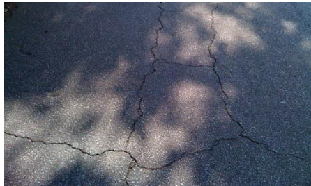
Gambar 2.10 Retak diagonal ( diagonal cracks ) (Sumber: Google Image )
