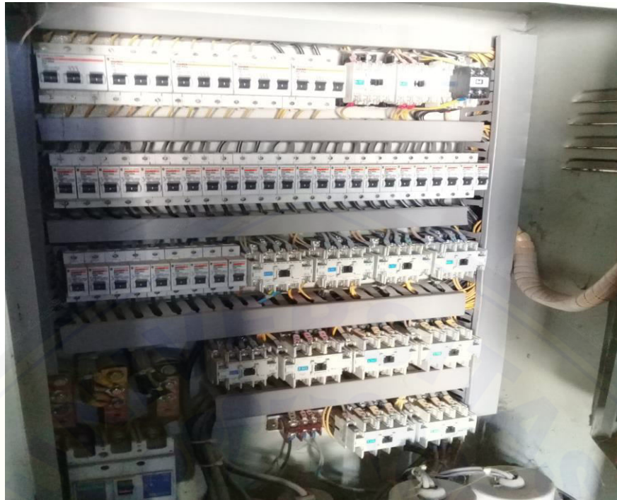
GAMBAR 1. INSTALASI KAPASITOR BANK
