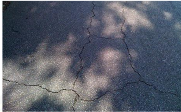
Gambar 2.3 Retak Halus ( hair cracking )
