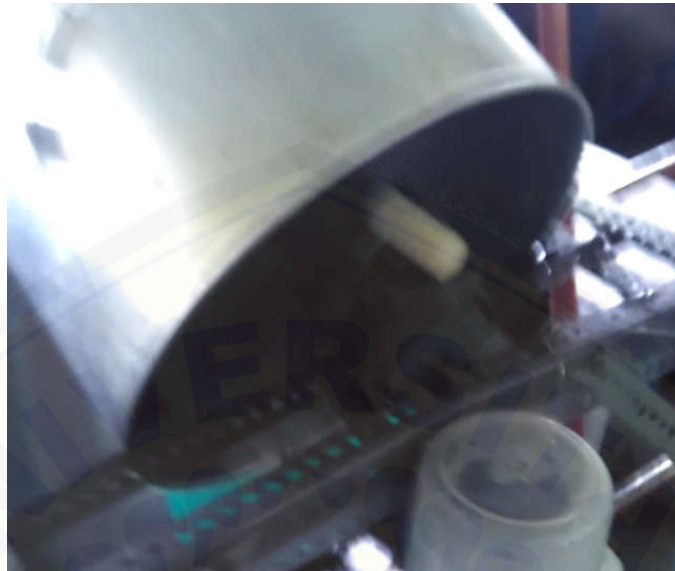
Gambar Kipas cooling tower
