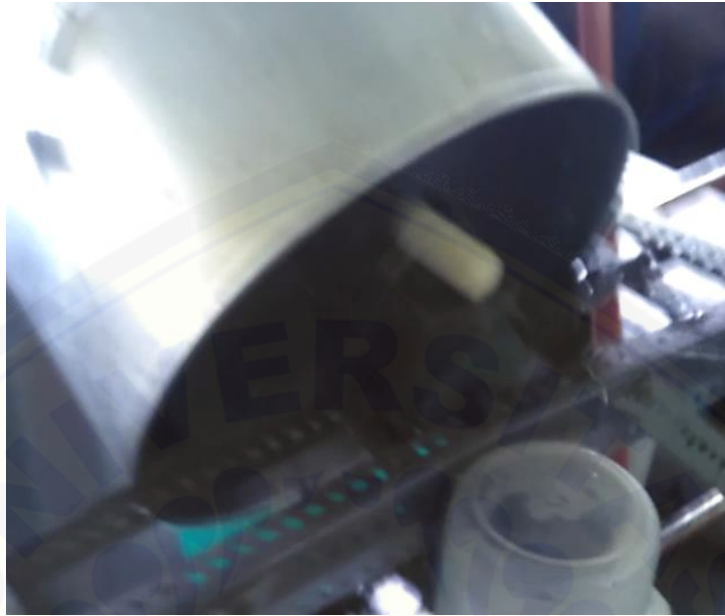
Gambar Kipas cooling tower
