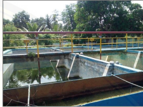
2. Bak Aerasi UPLC
