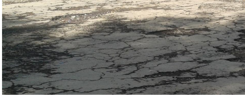
Gambar 2.14 Retak susut ( shrinkage cracks )
