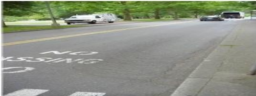
Gambar 2.15 Retak selip ( slippage cracks )
