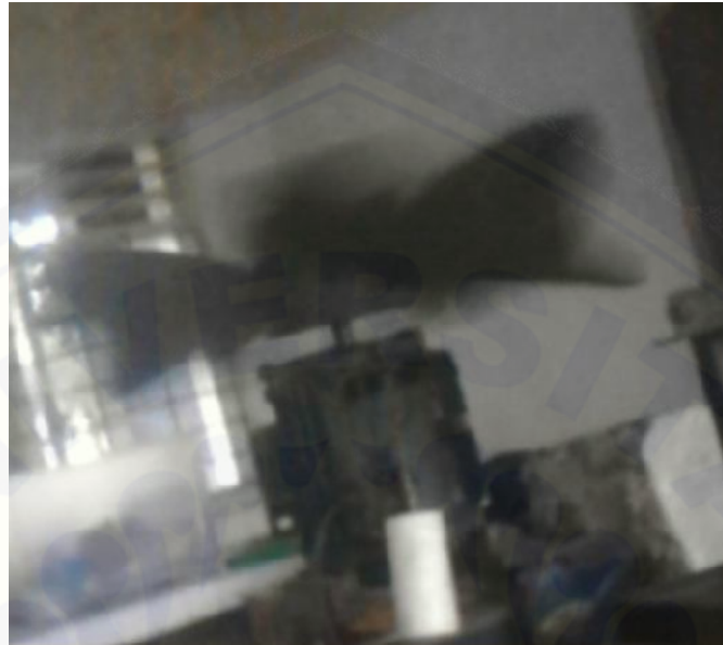
Gambar kipas cooling tower
