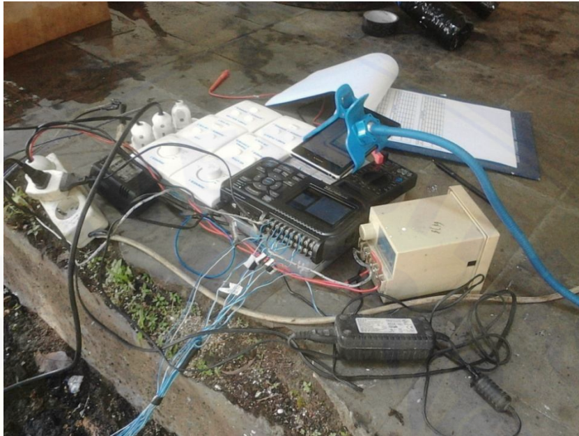
Gambar alat pengontrol cooling tower
