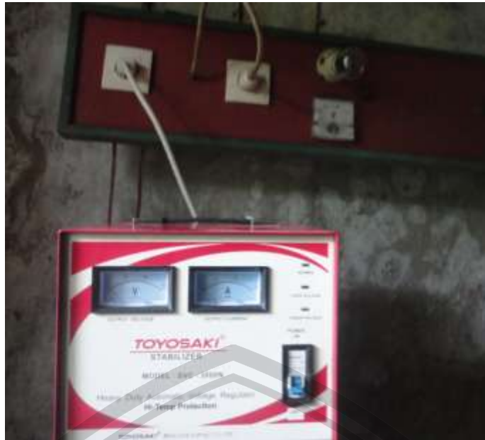
Unit penstabil tegangan AVR (Automatic Voltage Regulator)
