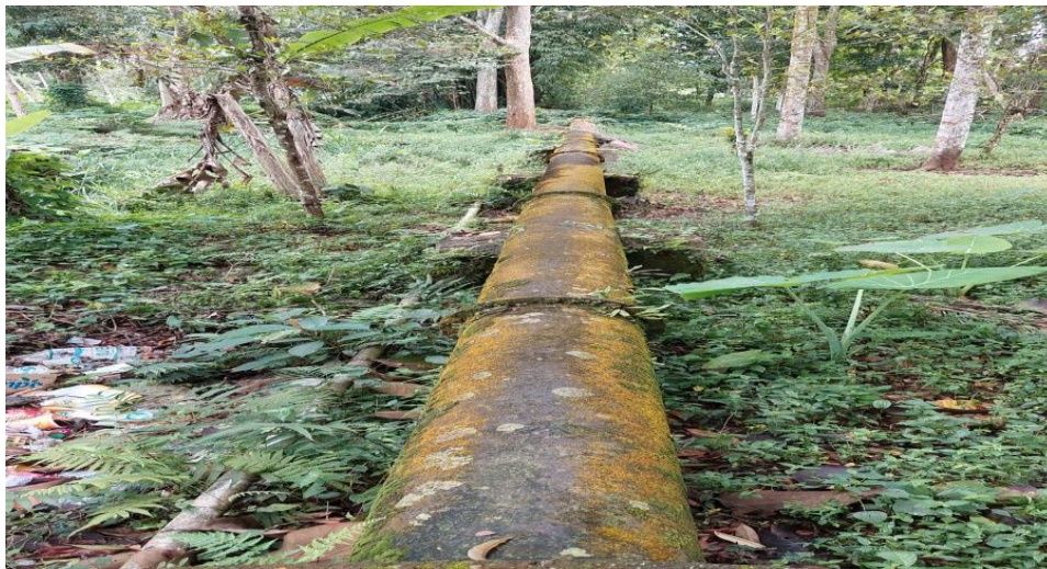
Gambar 4.1 Pipa Penstock PLTMh Sentool
