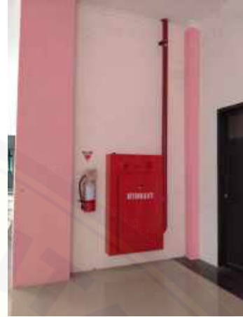
(b) Sistem Hydrant Lantai 2
