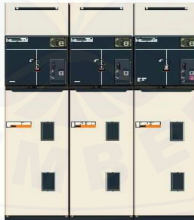
(c) Cubicle Set Gardu Distribusi
