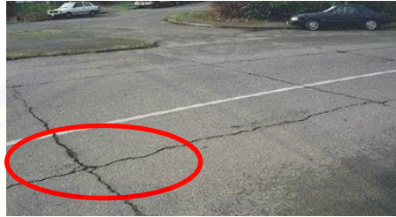
Gambar 2.5 Retak sambungan bahu dan perkerasan (Sumber: https://image.slidesharecdn.com/02aguskerusakanpadaperkerasanaspal )
