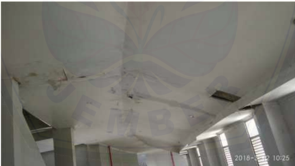
Lampiran 2. Kerusakan langit-langit
