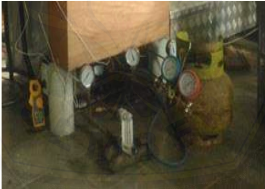
Gambar I.8 Proses Pengisian Refrigerant
