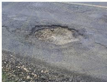
Gambar 2.18 Lubang ( potholes ) (Sumber: Google Images)
