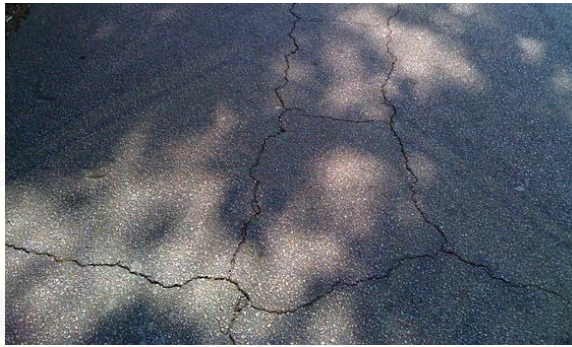
Gambar 2.4 Retak halus ( hair cracking ) (Sumber: Google Images)
