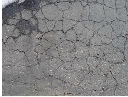
Gambar 2.11 Retak Susut ( shrinkage cracks ) (Sumber: Google Images)
