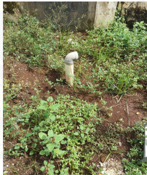
Septic tank Puskesmas
