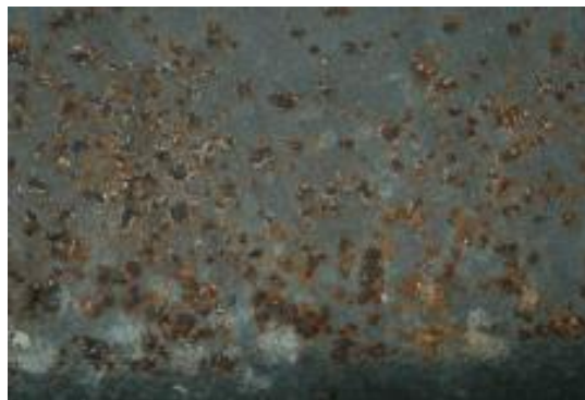
Gambar 2.4 Korosi Sumuran (Sumber: Utomo, 2009)
