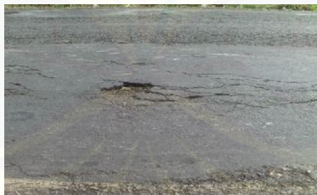
Gambar 2.2 Tambalan dan tambalan galian utilitas ( Patching and Utility Cut Patching ) (Sumber: Dokumentasi, 2014)
