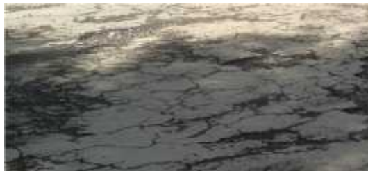
Gambar 2.9 Retak susut ( shrinkage cracks ) (Sumber : Sumantri, 2015)
