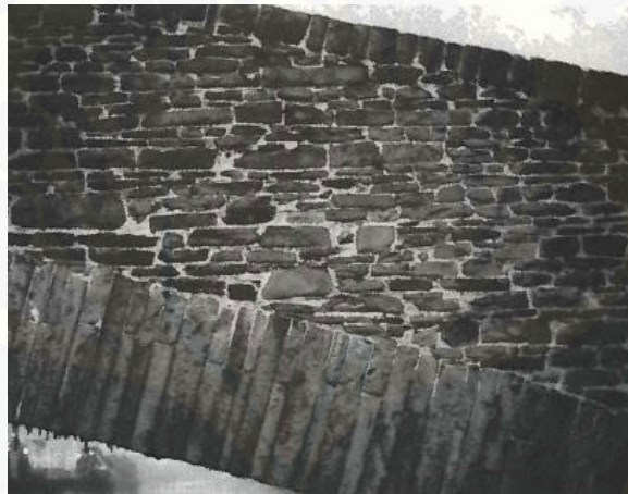
Gambar 2.3 Voussoir dan parapet pada Pontypridd (photographed by Ted Ruddock, reproduced by permission of Cambridge University Press) (Sumber: Jacques Heyman, 1982)
