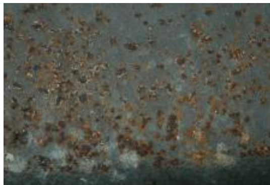
Gambar 2.4 Korosi Sumuran (Sumber: Utomo, 2009)
