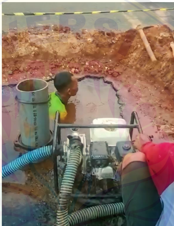
Gambar 1 Kerusakan Pipa Bocor HIPPAM
