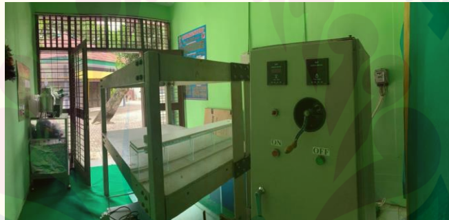
Gambar 3.2 Alat Current Transformeer (CT)
