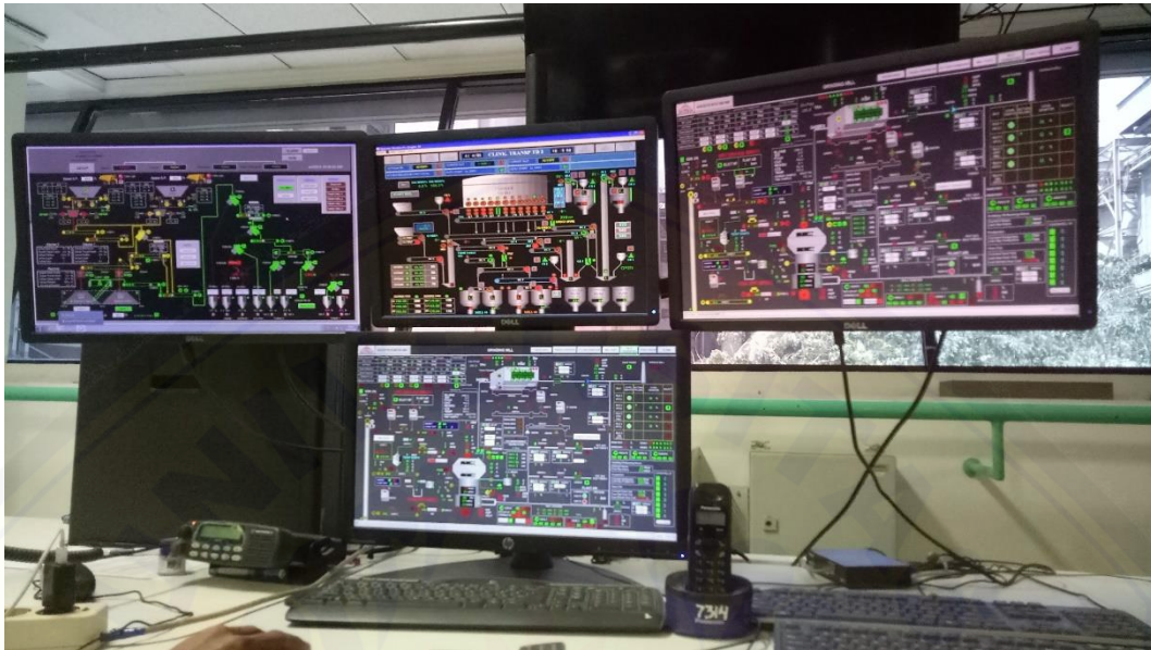
Lampiran 7 control room
