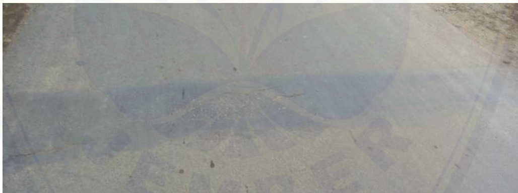
Gambar 2.12 Tambalan dan tambalan galian utilitas ( patching and utility cut patching )
