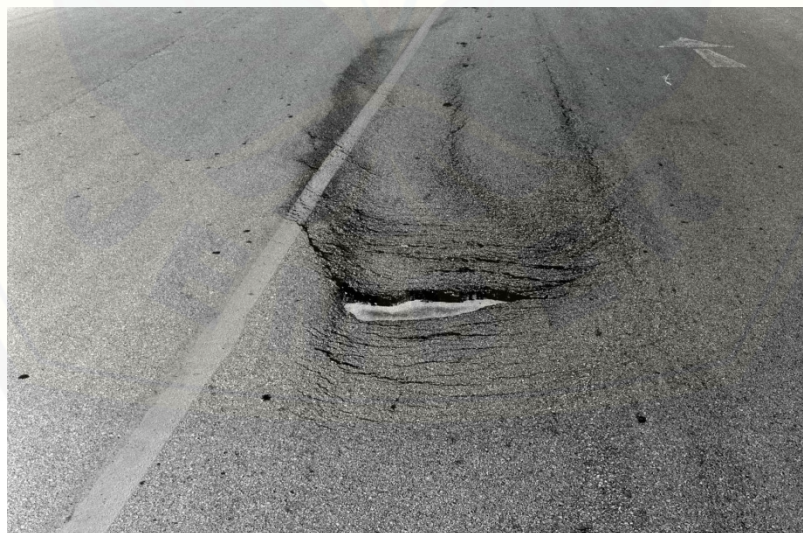
Gambar 2.18 Retak slip ( slippage cracking ) (Sumber: Google Images, 2017)
